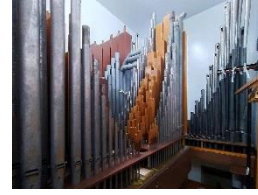
the new pipe organ chamber
