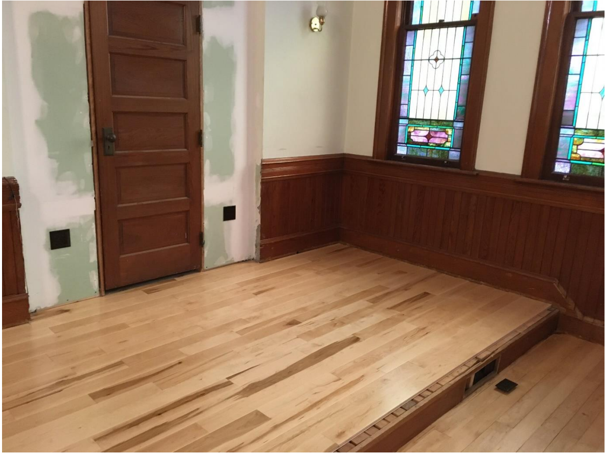
The new floor for the choir loft! The closet door is taken from the upstairs classroom closet. It matches pretty well!
